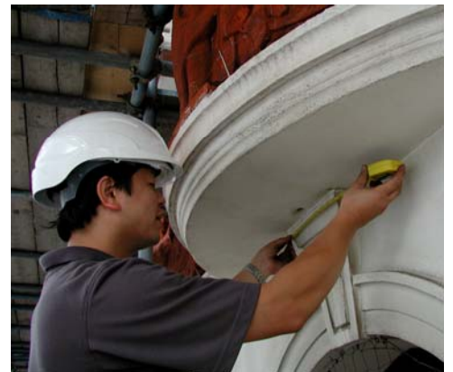
Assessment of a stone corbel
