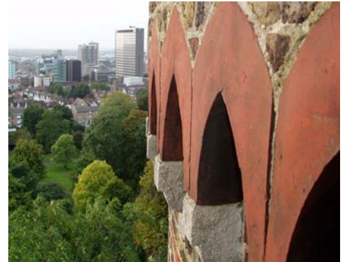
Condition of historic masonry
