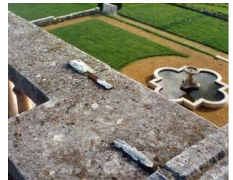
Lead coated metal fixings in old stonework
