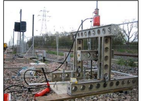
Pullout tests on M48 railway gantry anchor studs, including movement measurement. A proof load of 103kN was applied.
