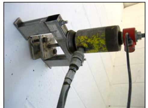
In situ pullout test on M12 self-tapping screw fixed into concrete column.
