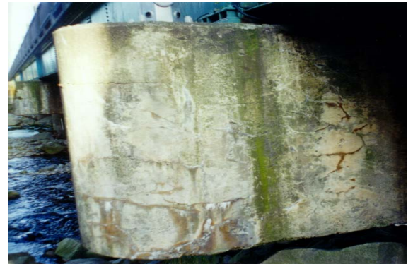
Alkali silica reaction in a bridge pier
