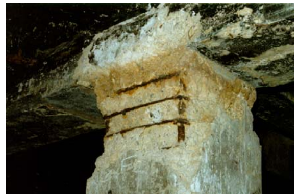
Frost attack in a cold store
